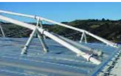
The roof is constructed with an ETFE sandwiched in an aluminium frame
