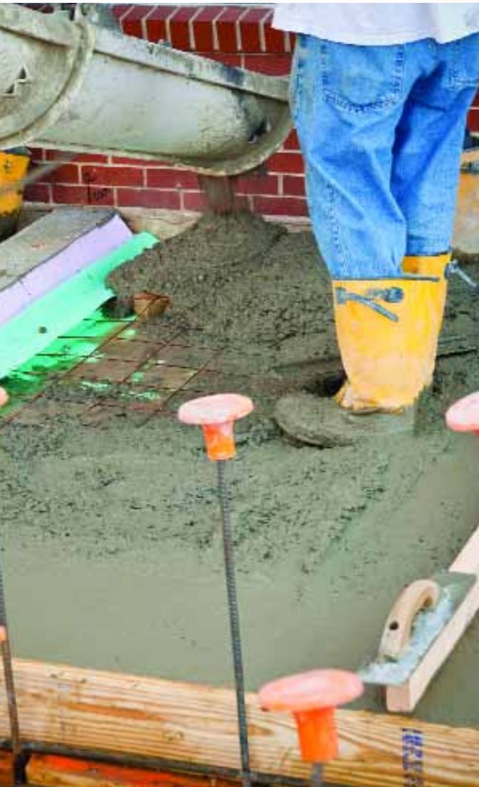
Sections of concrete shrink to leave a gap of anything up to 25mm wide between slabs
